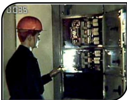
** With ABB TVOC-2 Arc Guard protection
